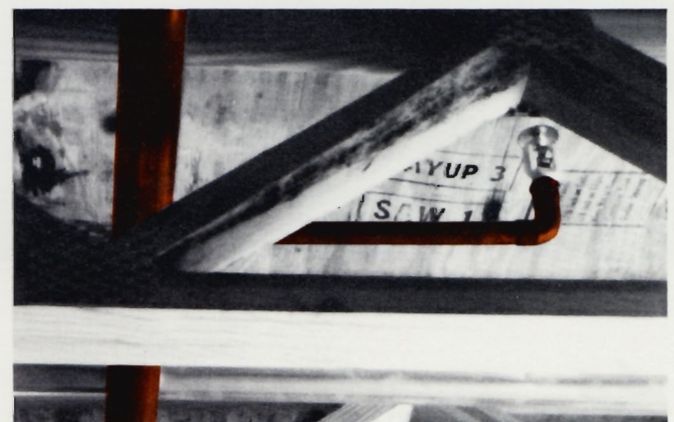
Figure 5: Typical attic upright head.
