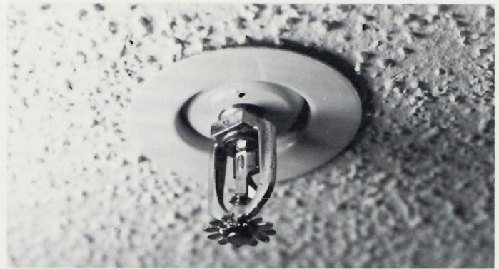
Figure 6: Typical ceiling pendent.
